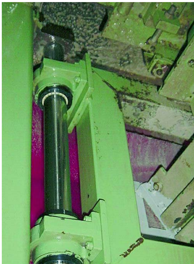
Picture PM0805-02: Haas Maschinenbau, Oberbrück Concrete pipe mortising machine in mud: since ball bushes didn't work, Haas Maschinenbau (Oberbrück) replaced these with the DryLin linear guide system from igus. The machine has now been running without any problems whatsoever for three years.
